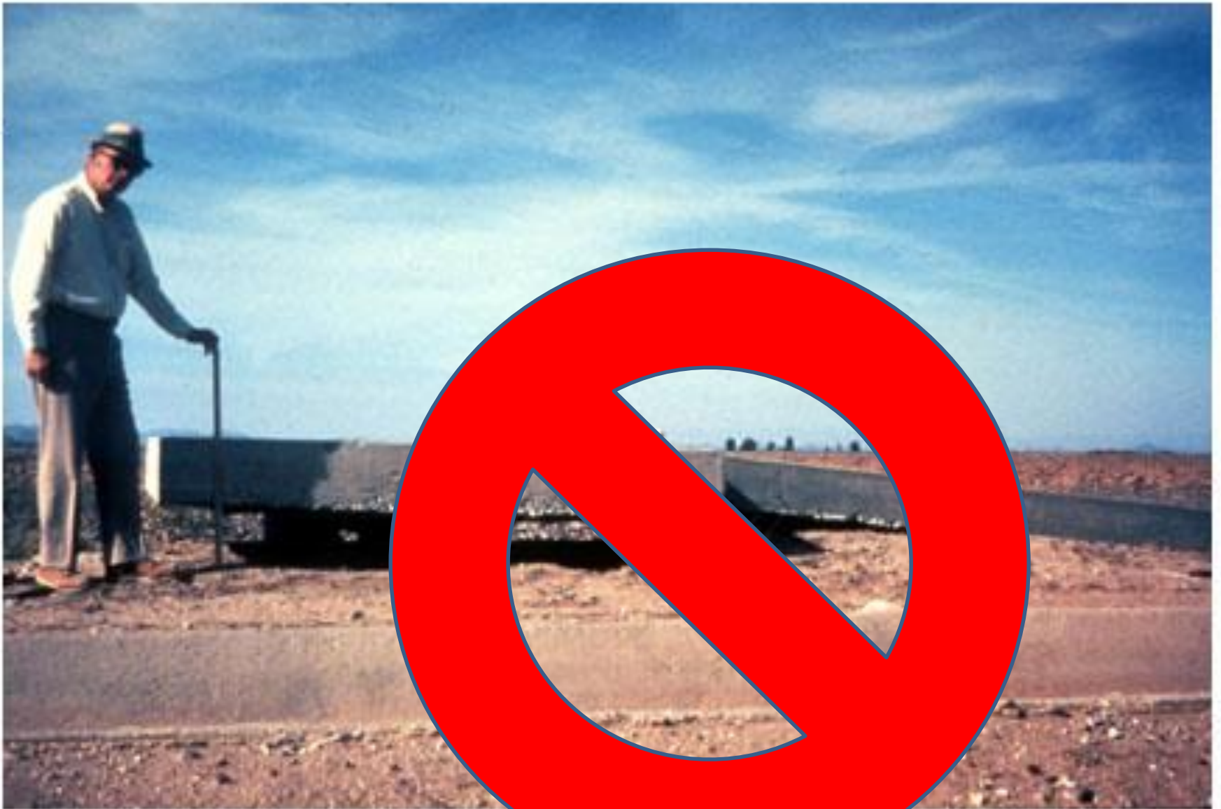
Figure 3. Visible effect of subsidence on land surface. Concrete pad on well casing was originally at land surface. The rigid well casing has not sunk along with the land surface.
